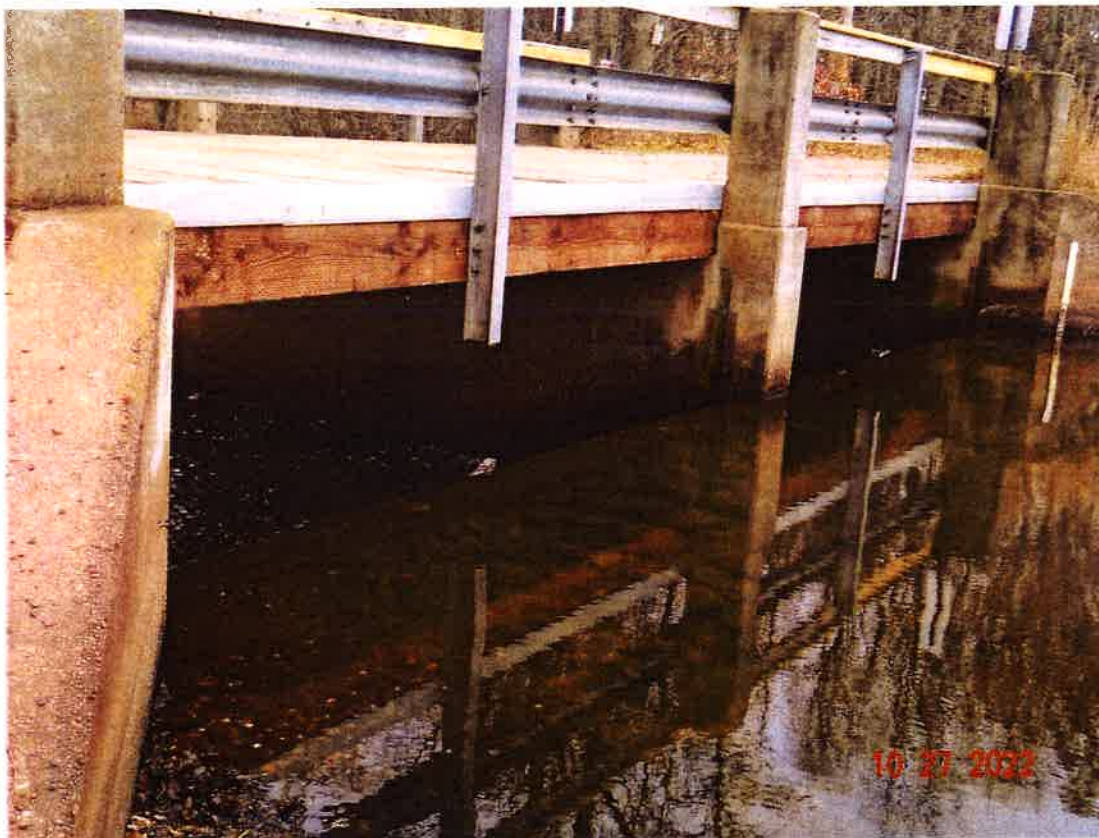
Overview of Upstream side of dam. Small amount of concrete degradation around pier and abutments.
