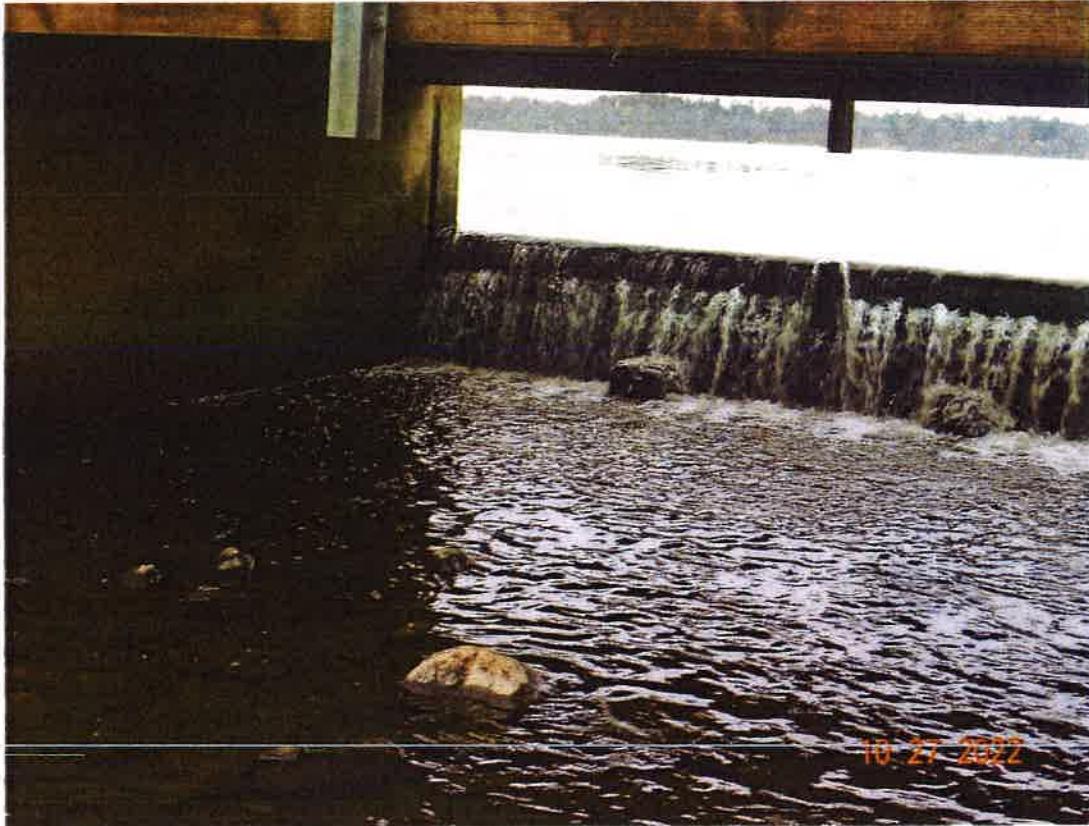
Looking upstream at dam, higher flows than last year could not see leak.
