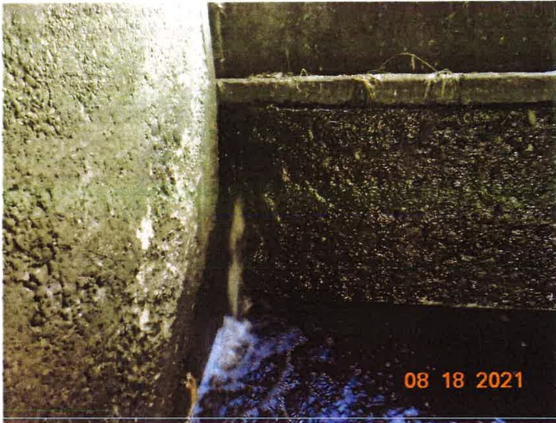
Photo of leaking between concrete weir and concrete abutment during drought of 2021.
