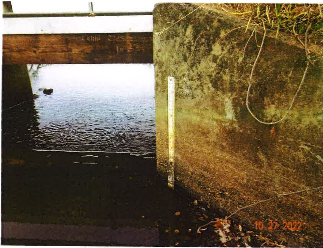
Gage and concrete degradation.
