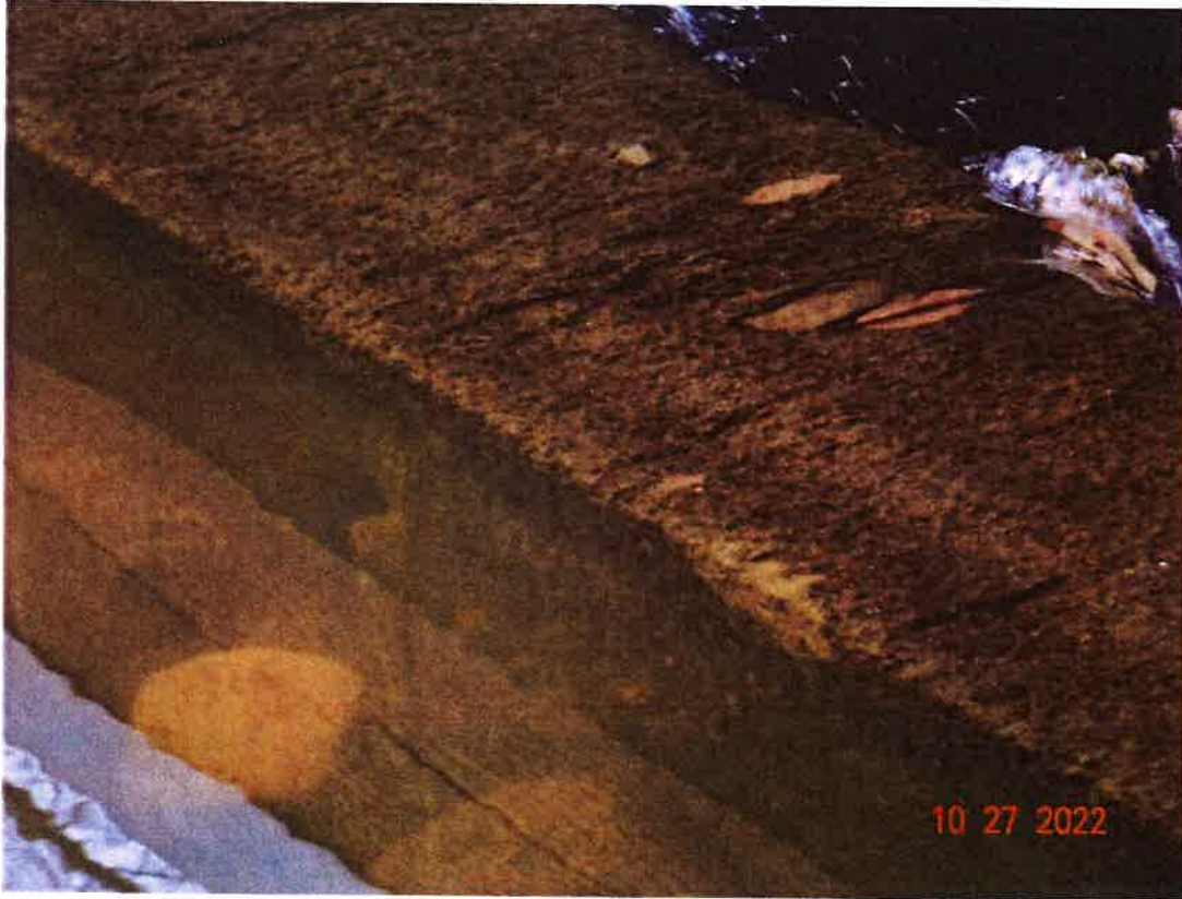
Concrete weir, showing erosion.
