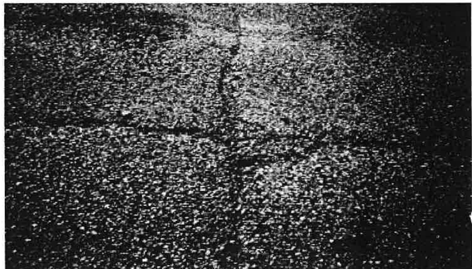
▶ Open and raveled block cracks.
