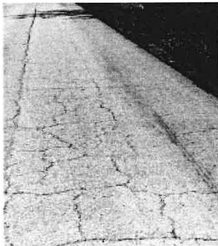
▲ Extensive block cracking in an irregular pattern.
