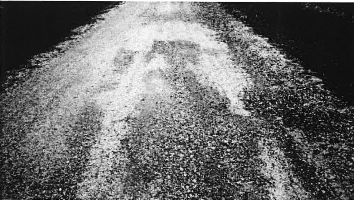
◀ Extensive loss of surface. Rebuild.
