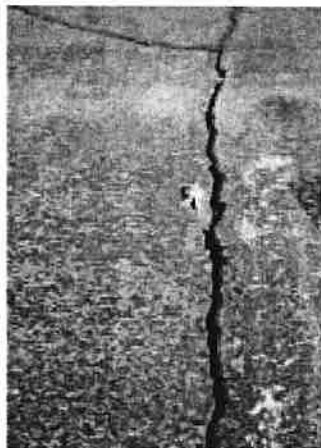
▲ Open crack – 1/2" or more in width.
