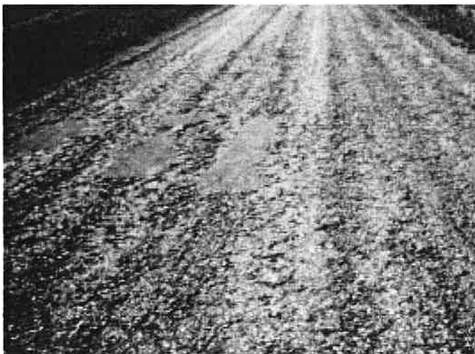
◀ Severe raveling and loss of surface material.
