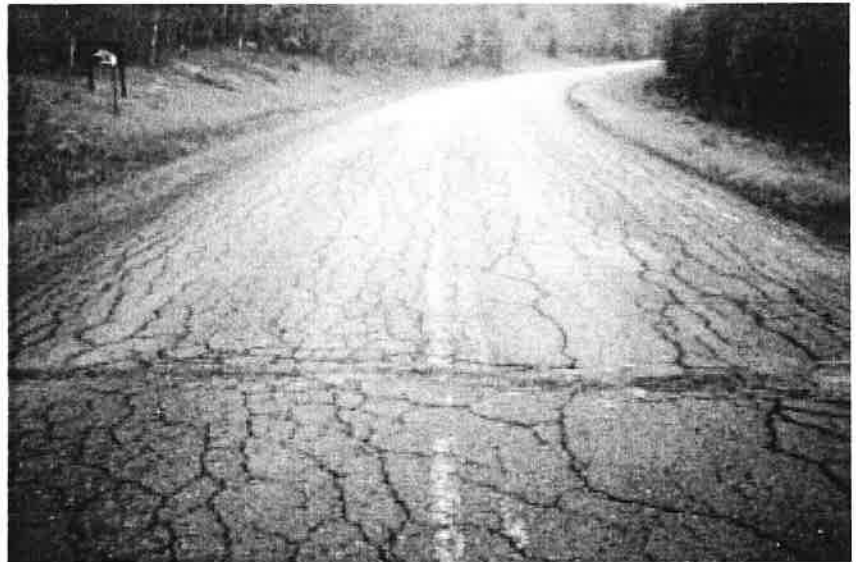
▶ Extensive alligator cracking. Pulverize and rebuild.
