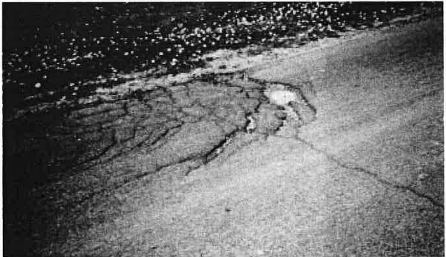
► Crescent-shaped cracks characteristic of slippage.
