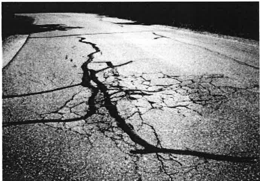
► Frost heave damage from spring break-up.
