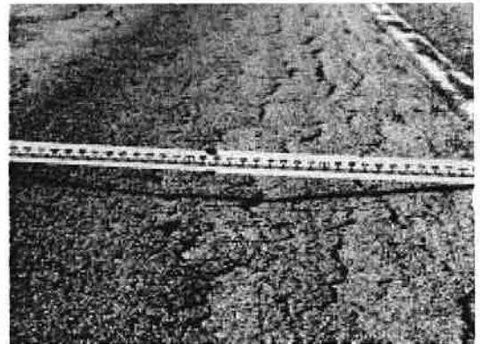
▲ Severe rutting. Strengthen base and reconstruct.
