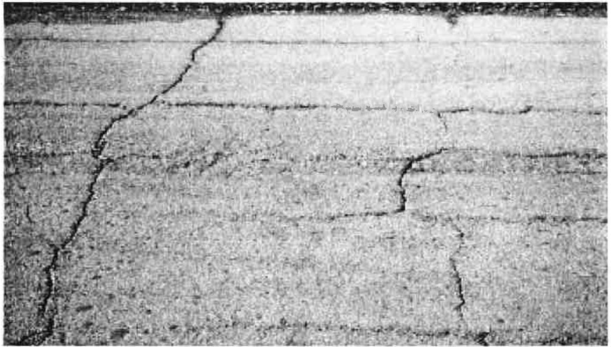
▼ Block cracking with open cracks.
