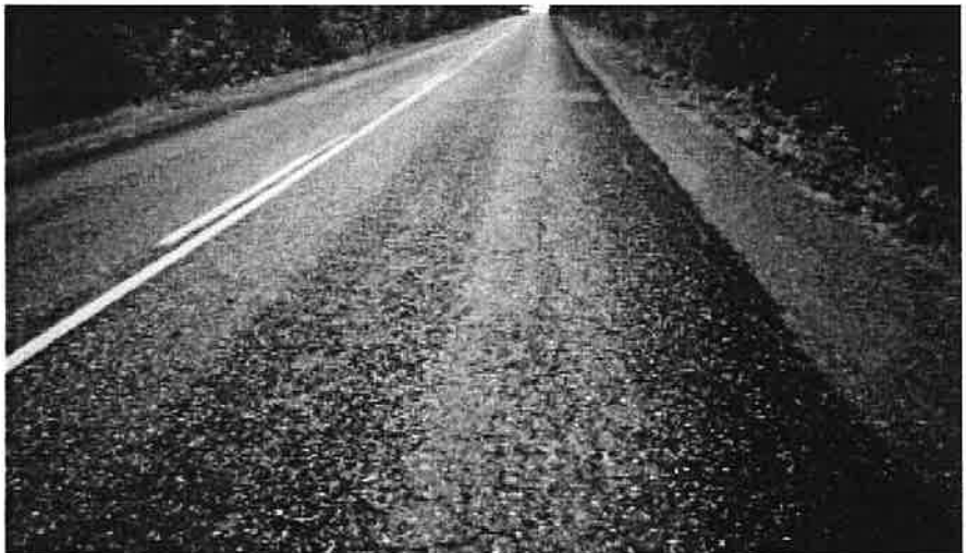
► Moderate to severe raveling in wheel paths.
