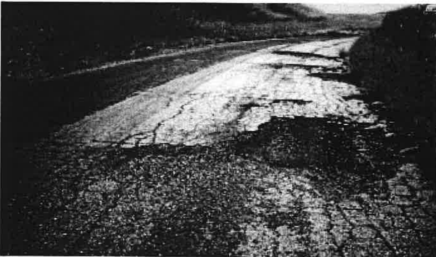
◀ Potholes and severe alligator cracking. Failed pavement. Reconstruct.
