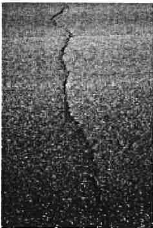
▲ Tight cracks less than 1/4" in width.
