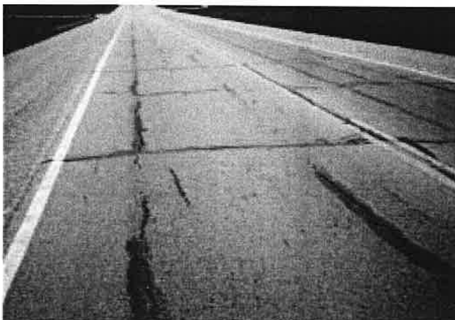
▼ Load-related cracks in wheel path plus centerline cracking.
