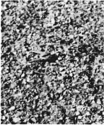
Severe raveling with ▼ extreme loss of aggregate.
