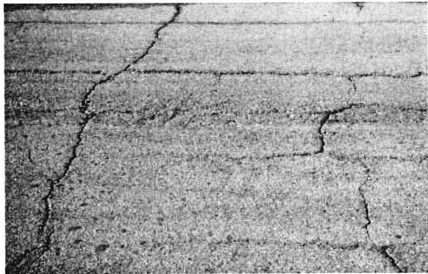
▶ Intermediate-size block cracking, 1'-5' across with open cracks.
