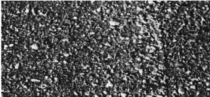
◀ Moderate to severe raveling. Erosion further exposes large aggregate.
