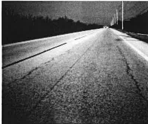
Load cracking and slight ▼ rutting in wheel path.
