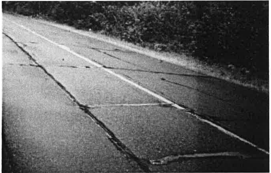
► Concrete joints reflected through bituminous overlay.
