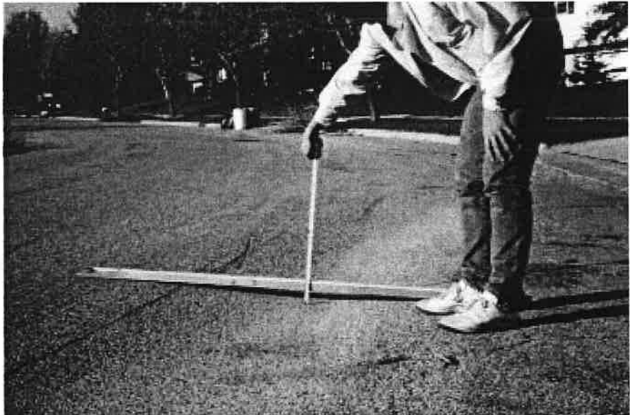
► Severe settling from utility trench.
