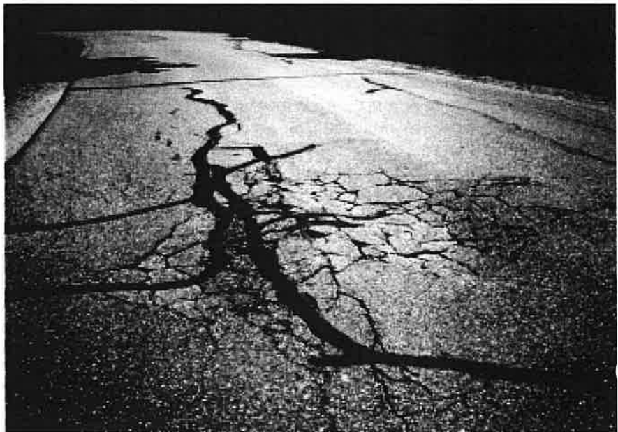
► Frost heave damage from spring break-up.
