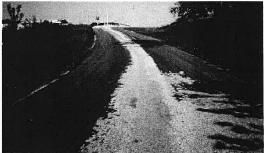
► Edge wedging. Pavement edges strengthened with wedges of asphalt. Patch is in very good condition.
