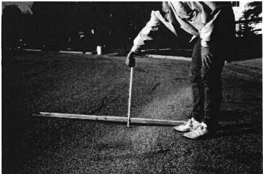
► Severe settling from utility trench.
