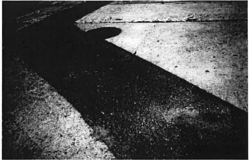
► Typical repair of utility excavation. Patch in fair to good condition.
