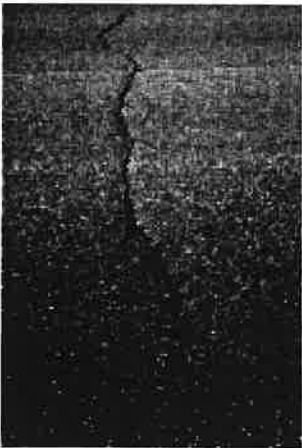
▲ Tight cracks less than 1/4" in width.
