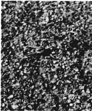
Severe raveling with ▼ extreme loss of aggregate.
