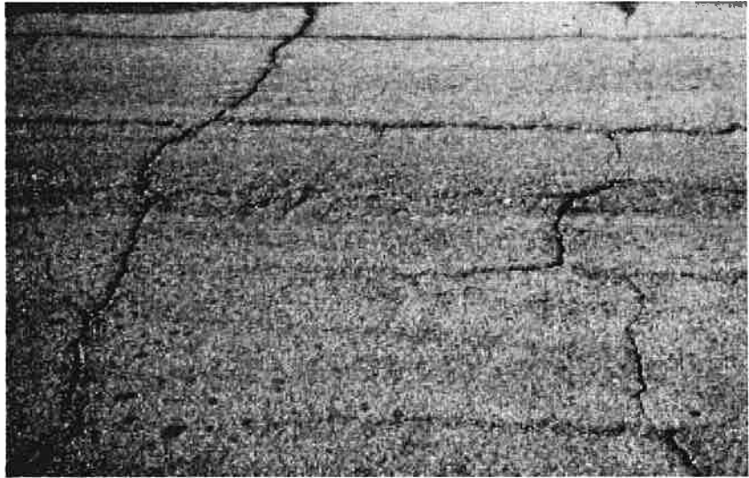
▶ Intermediate-size block cracking, 1'-5' across with open cracks.
