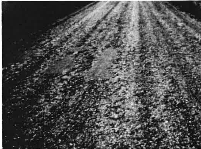
◀ Severe raveling and loss of surface material.
