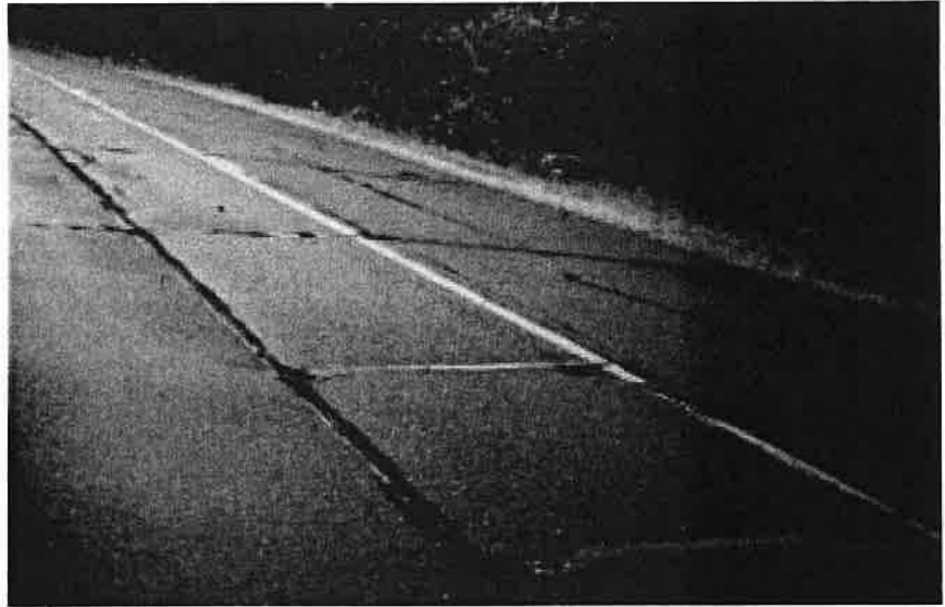
► Concrete joints reflected through bituminous overlay.
