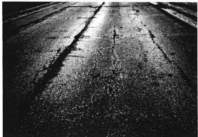
Multiple open cracks at open line, wheelpaths and lane center. ▼
