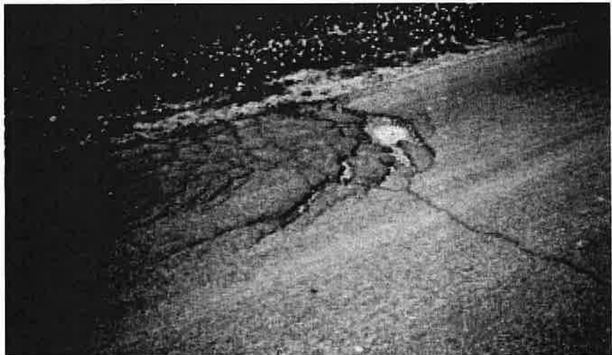
► Crescent-shaped cracks characteristic of slippage.
