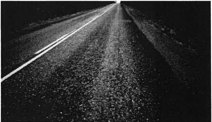
► Moderate to severe raveling in wheel paths.
