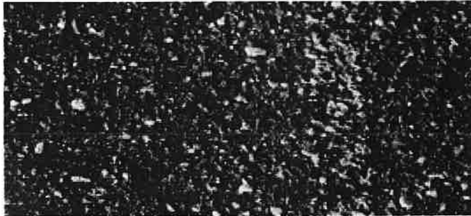
◀ Moderate to severe raveling. Erosion further exposes large aggregate.
