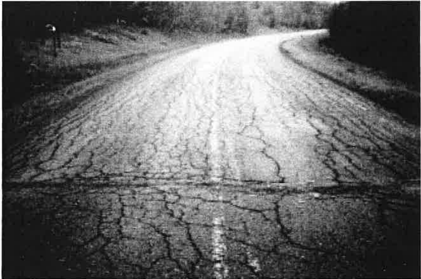
▶ Extensive alligator cracking. Pulverize and rebuild.
