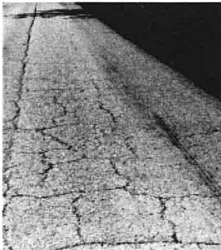
▲ Extensive block cracking in an irregular pattern.
