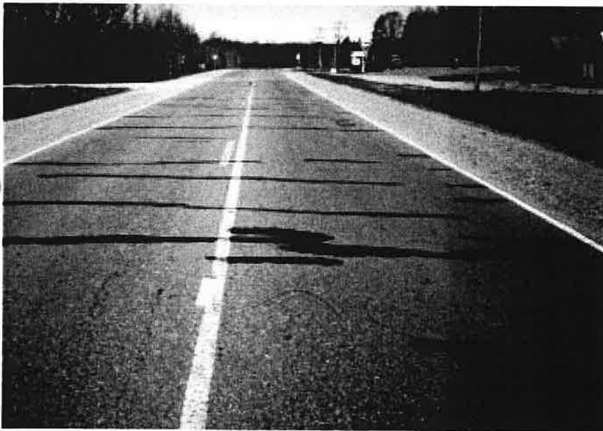
◀ Sealed cracks, a few feet apart.
