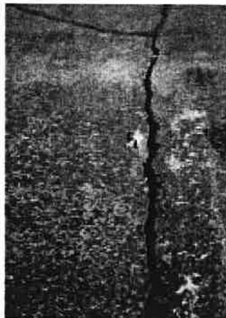
▲ Open crack — 1/2" or more in width.
