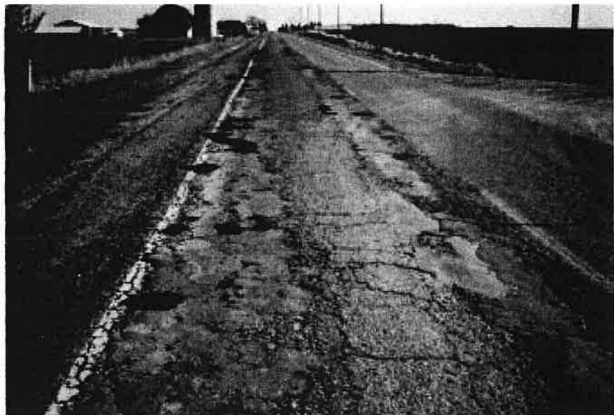
► Extensive patching in very poor condition.
