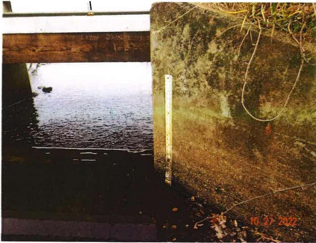
Gage and concrete degradation.
