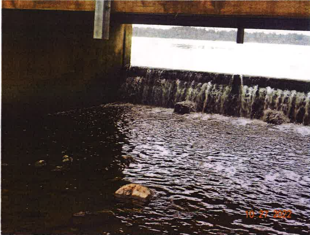
Looking upstream at dam, higher flows than last year could not see leak.
