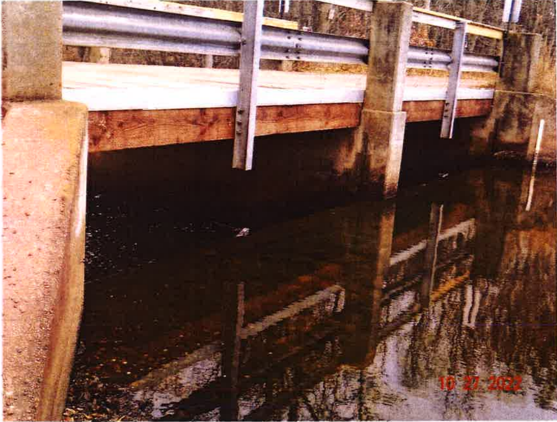
Overview of Upstream side of dam. Small amount of concrete degradation around pier and abutments.
