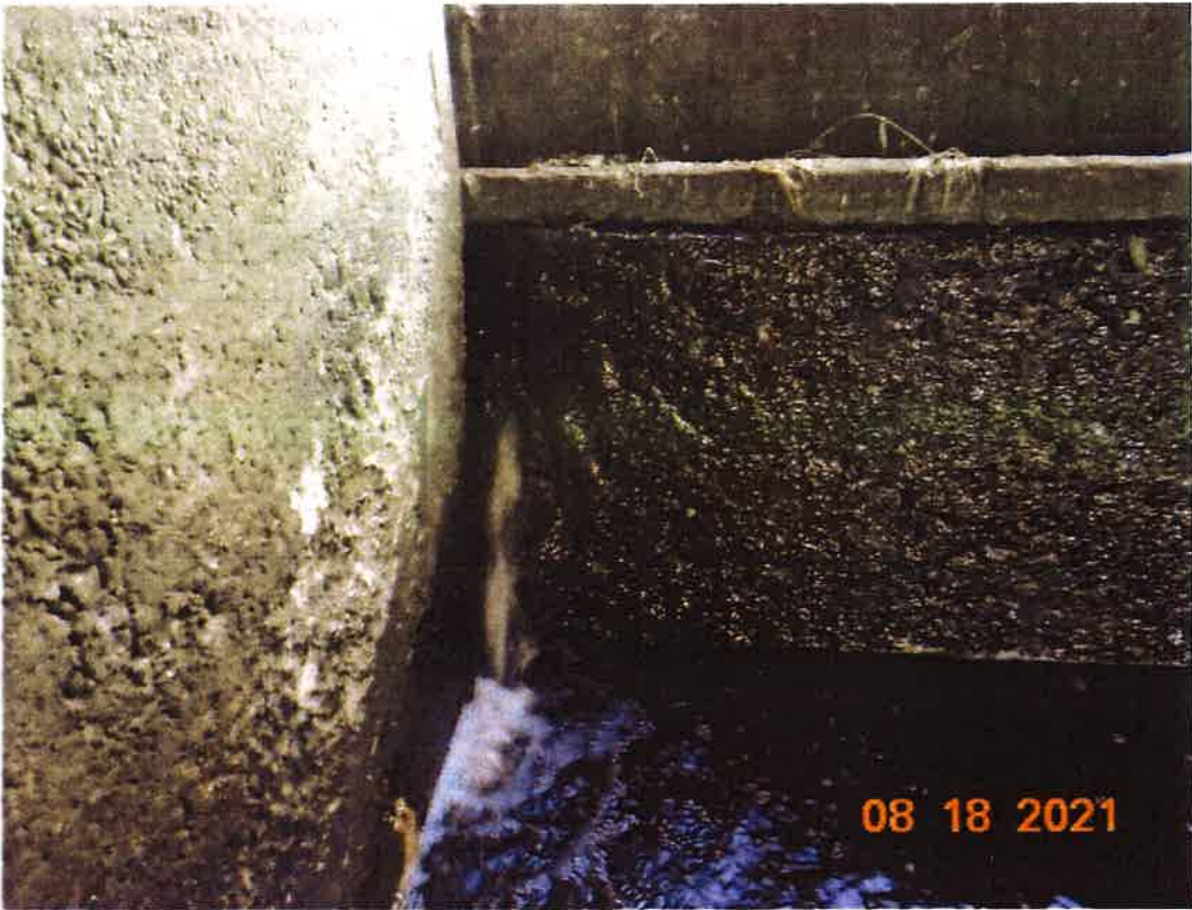
Photo of leaking between concrete weir and concrete abutment during drought of 2021.
