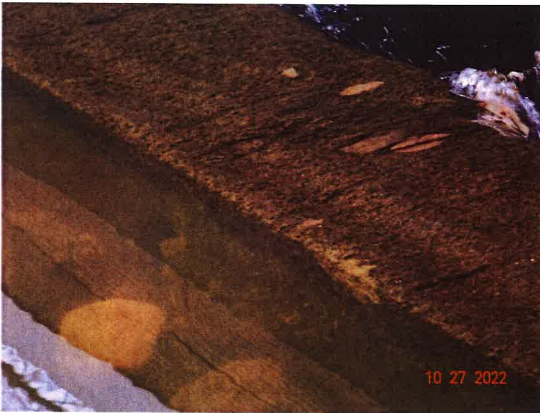
Concrete weir, showing erosion.
